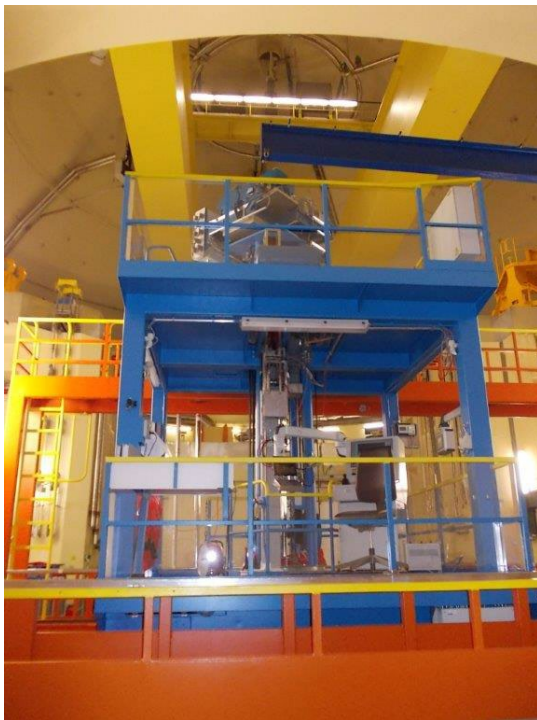
Refueling machine at Borssele NPP, Netherlands
