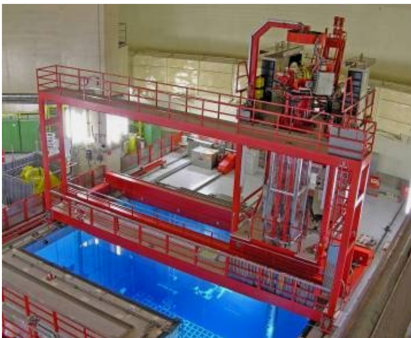
Refueling machine at Biblis NPP, Germany
