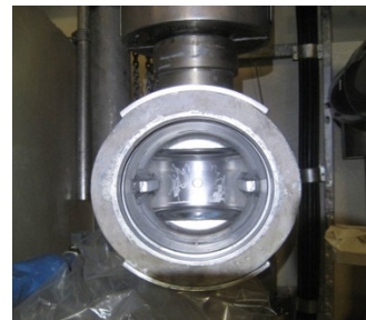
Open valve of a volume control system after decontamination
