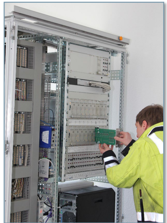
STUDIS-SE permanent installation
