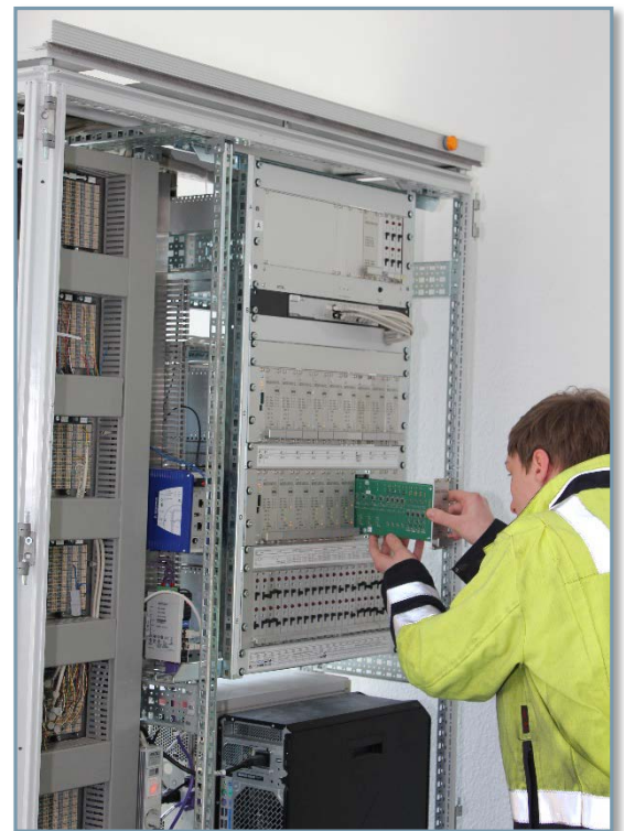
STUDIS-SE permanent installation
