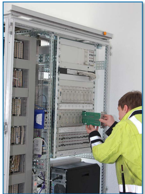
STUDIS-SE Installation Leittechnik-Raum
